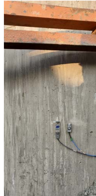
Fig. 7. Close-up view of accelerometer and strain gauge installed on a 1500 mm diameter pile
